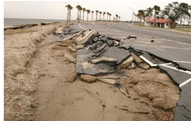
Figure 11.15d: Wave attack has undercut this coastal road.
